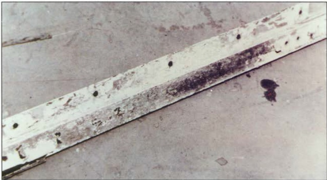
Figure 2-3. Uniform Etch Corrosion
